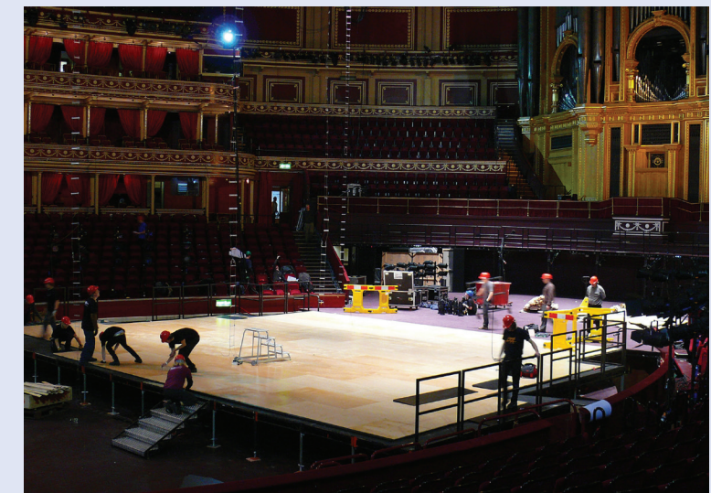
Harlequin Liberty® floor installation at the Royal Albert Hall. Panels had to be cut on-site to accommodate the iconic elliptical curve of the stage.
